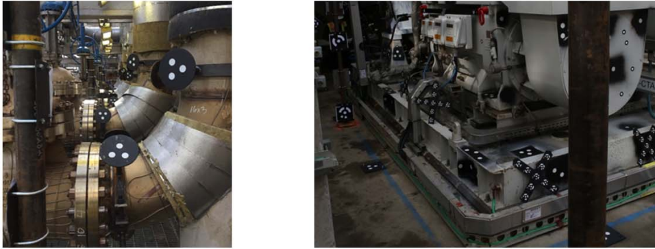
Figure 3 - Target dots seen on key equipment and piping. Picture on left shows the Suction/Discharge lines, where the largest piping displacements were seen. Picture on right, shows Pump C motor and baseplate with photogrammetry targets.
